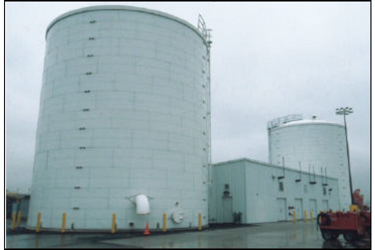
Pictured here are the water storage tanks used in the fire protection system for the new aircraft repair hangar at Wayne County Airport.
